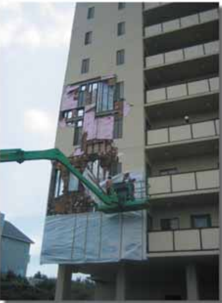
Windward Dunes Salter Path NC Damage from Hurricane Ophelia
